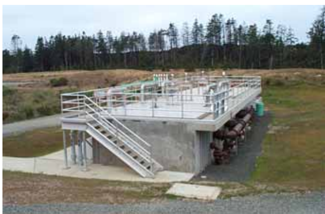
Fig. 5 Oversea MBR Installation for Land Irrigation
